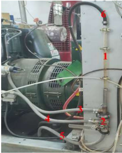
Figure 2 : Diesel flow meter
